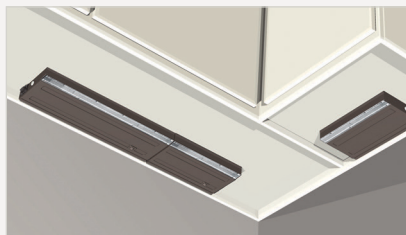
Back of Cabinet Installation – Direct wire connect.
